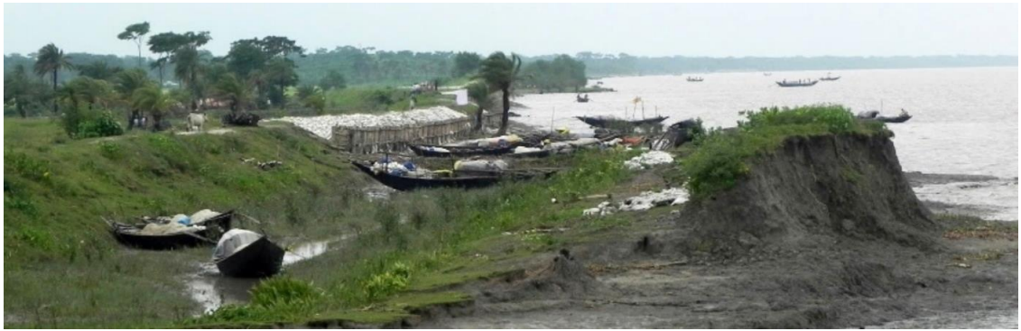
Photo-2: Damage by Cyclone Sidr on Polder 35/1 on Baleswar River
