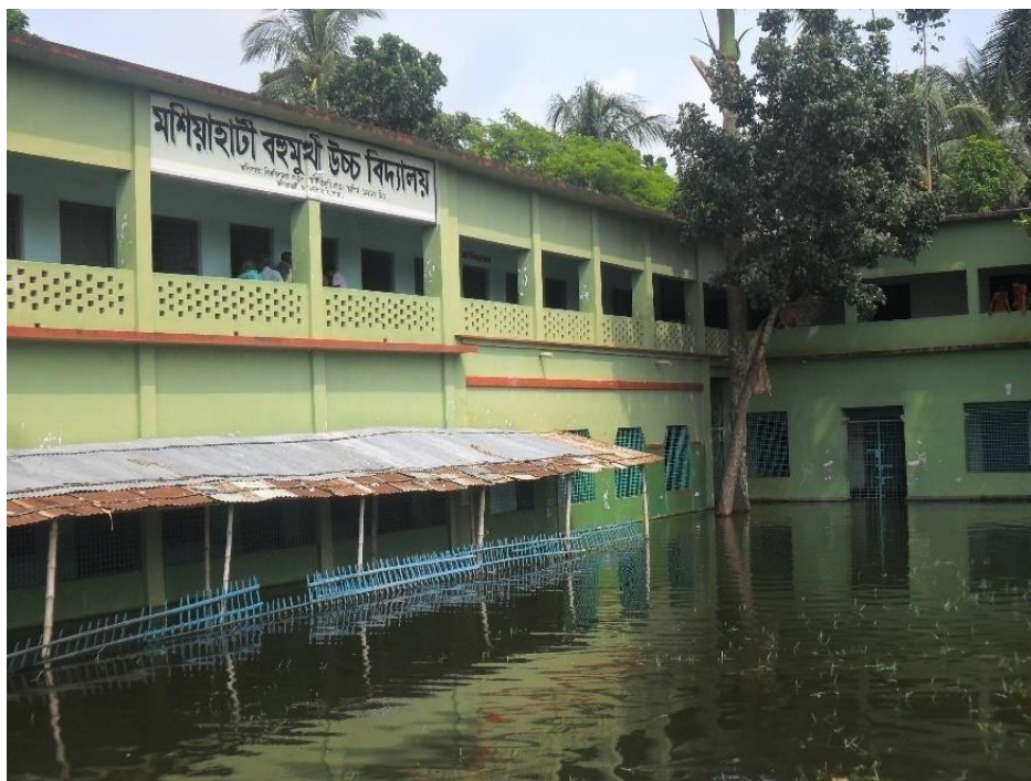
Photo-5: Drainage Congestion in Mosihati School (Polder-24) during September 2016
