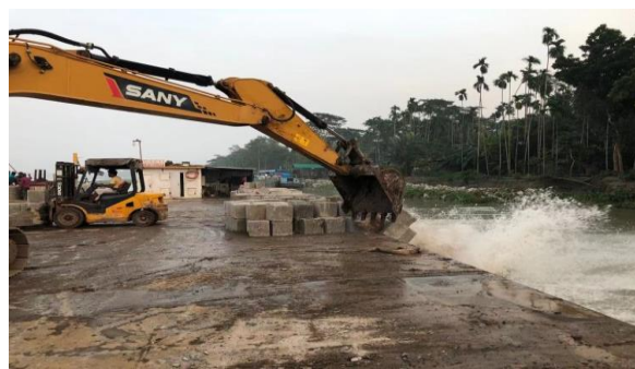
Figure 3-58: Dumping CC Block for river bank protection work (KM51+041-53+418) in Polder 39-2C
